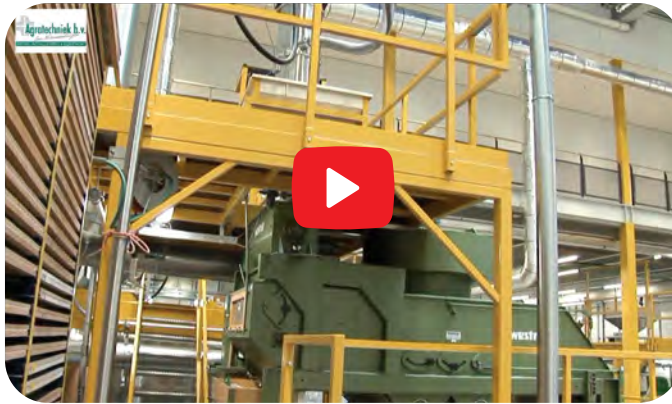
Watch exactly how a pneumatic vacuum conveying system automatically transfers seeds from floor level up and into a hopper for fast, efficient bag filling.
