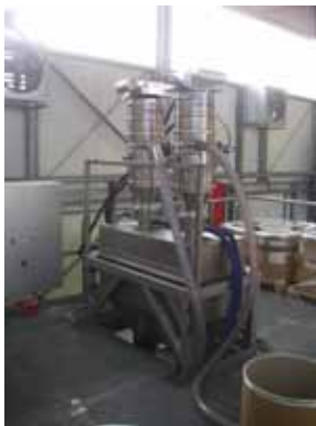
Figure 2: Two Vacuum Conveyors transfer different powders onto a powder processing/ production line; for the conveying pipeline here hoses were chosen.
